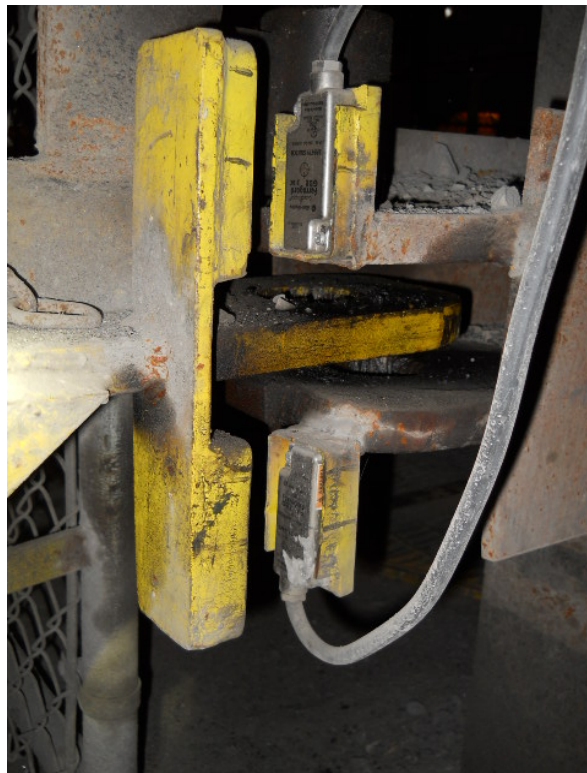
New Safety Switch Actuators Required by MSHA (post accident) Installed with Tamper Proof Bolts
