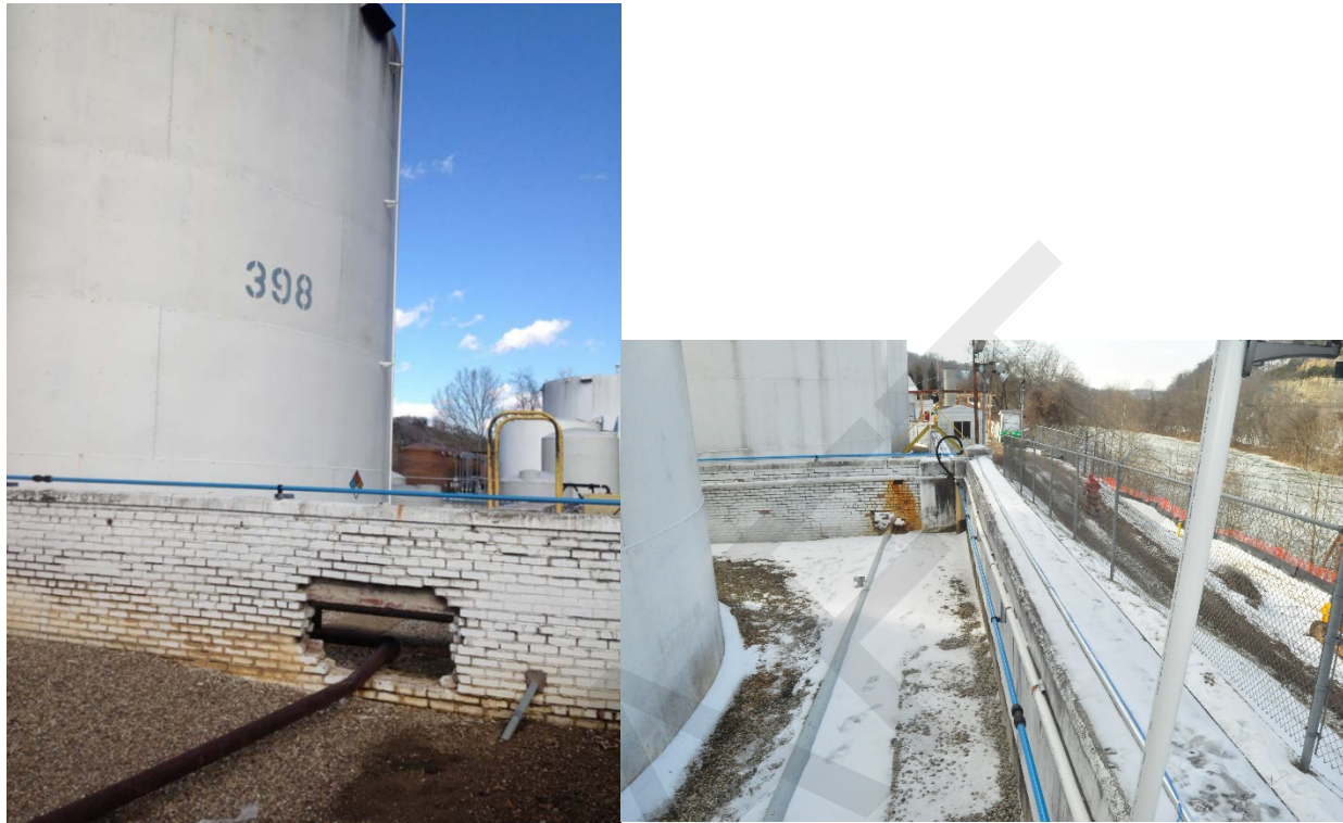
Figure 24. The dike walls that surrounded the tank farms were in poor condition. (Source: CSB)
