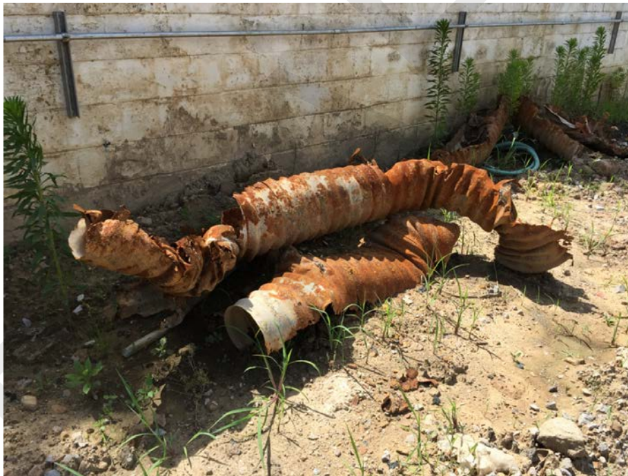
Figure 28. Photo taken on June 15, 2015, of remnants of the culvert that ran between tanks 394 and 395 beneath the site. (Source: CSB)
