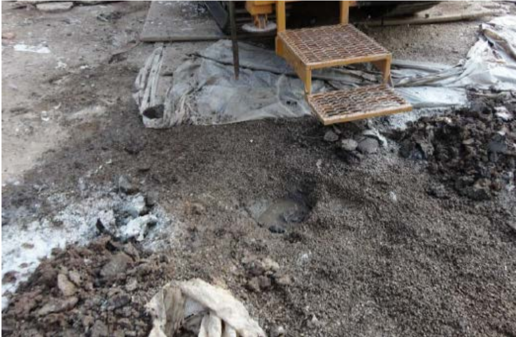
Figure 20. Gravel base under tank 396 and other MCHM tanks. (Source: Terracon)
