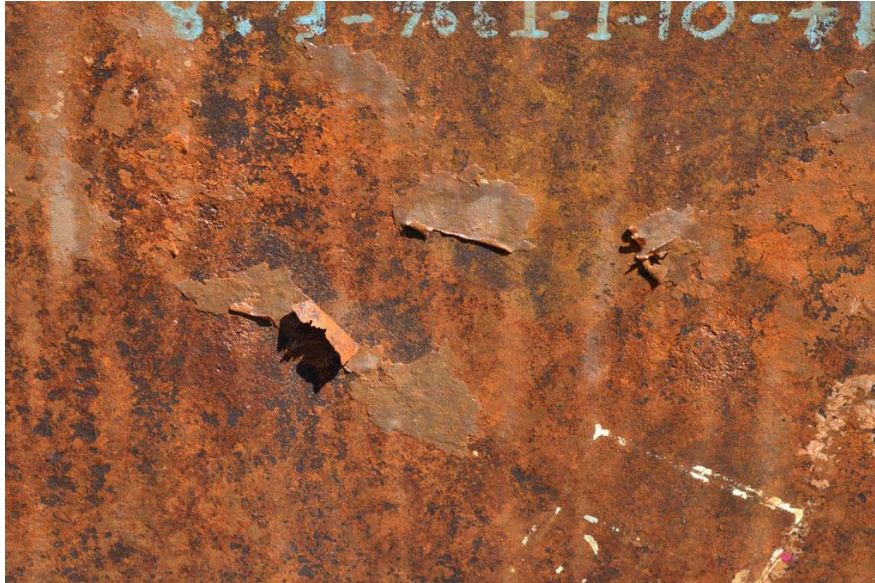
Figure 18. Remnants of coating on interior tank floor. (Source: CSB)
