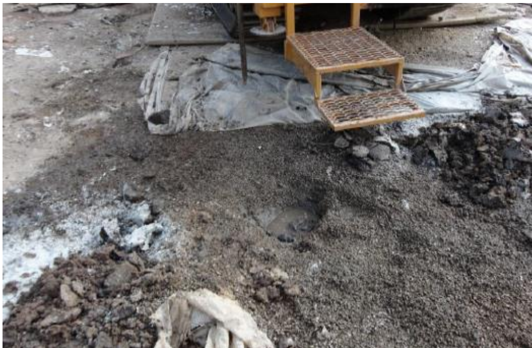
Figure 20. Gravel base under tank 396 and other tanks containing mixtures with Crude MCHM and PPH, Stripped. (Source: Terracon)
