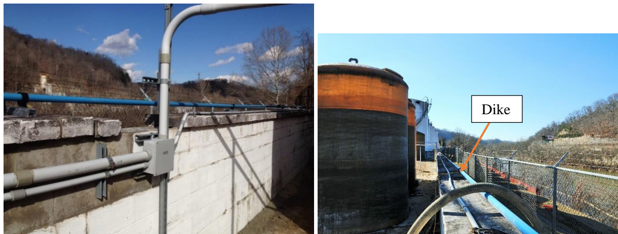
Figure 23. View from inside the dike wall facing the Elk River of the concrete block walls with no reinforcement (Left); dike wall along the tank farm parallel to the Elk River (Right). (Source: CSB)
