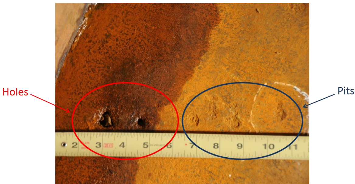
Figure 13. The bottom of tank 396 with holes and pits identified. (Source: CSB)
