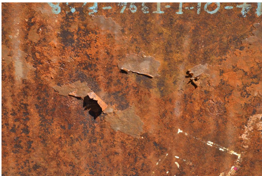
Figure 18. Remnants of coating on interior tank floor. (Source: Anamet 122 )
