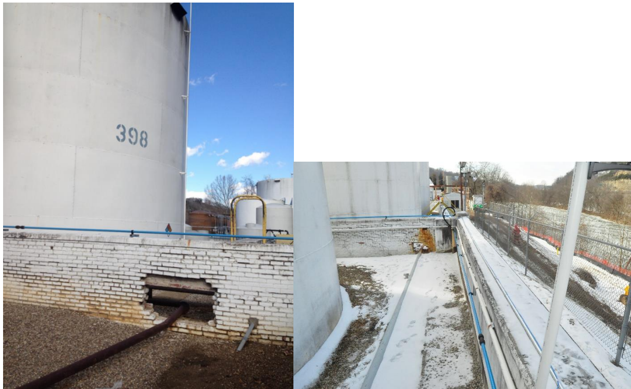
Figure 24. The dike walls that surrounded the tank farms were in poor condition. (Source: CSB)
