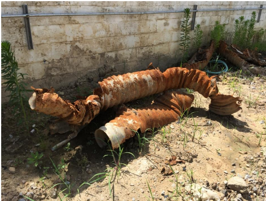
Figure 28. Photo taken on June 15, 2015, of remnants of the culvert that ran between tanks 394 and 395 beneath the site. (Source: CSB)
