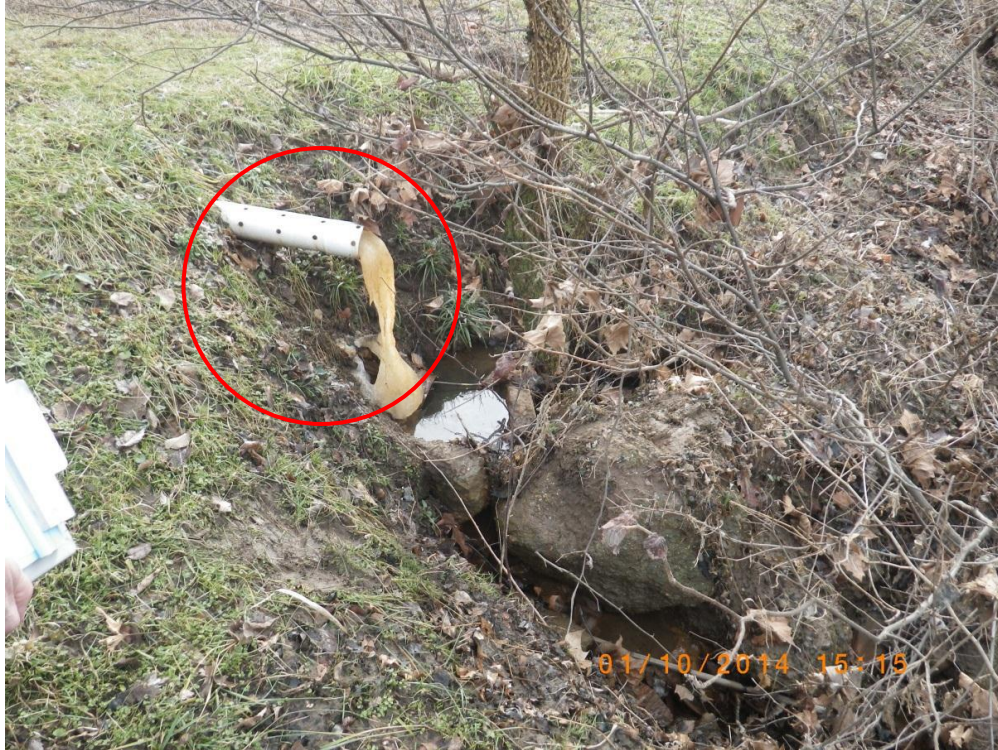
Figure 25. Ice-filled oil/water separator discharge pipe into the Elk River. (Source: WVDEP)
