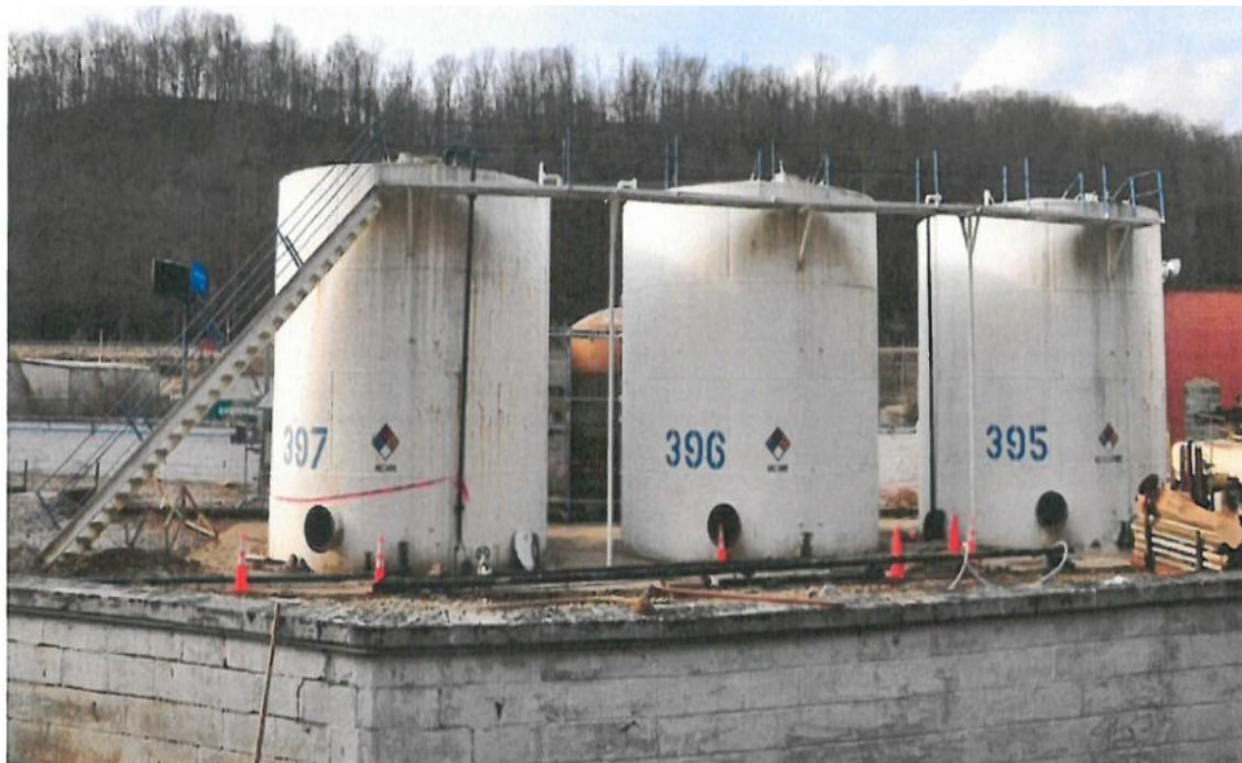
Figure 4. MCHM- and PPH, stripped-containing tanks at Freedom post-incident. (Source: CSB)
